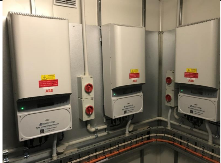
Grid-tie inverters 3 x ABB PVI-6000
