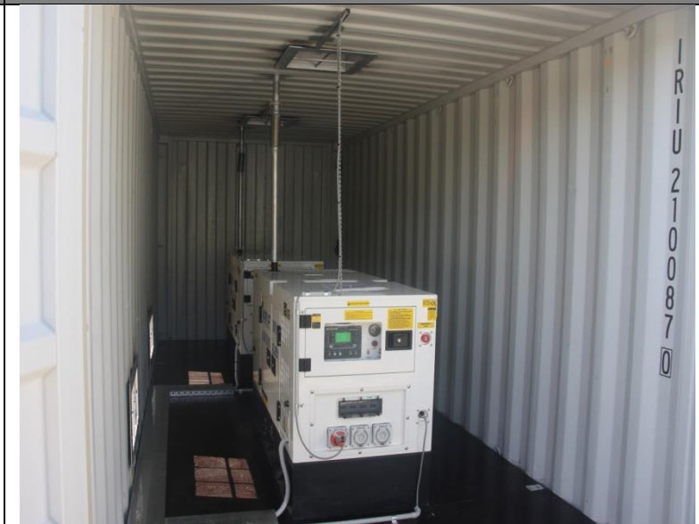
Diesel generator room
