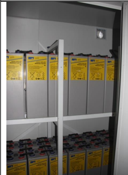
Battery bank & custom built stand
